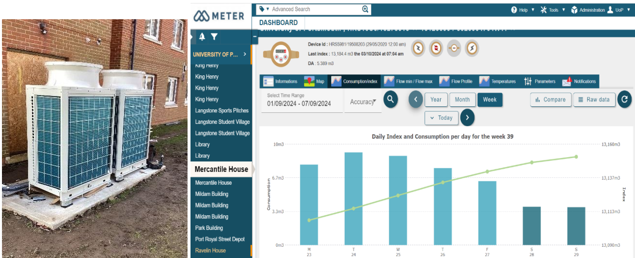
Air source heat technology at Langstone Campus. Monitoring water consumption online.
